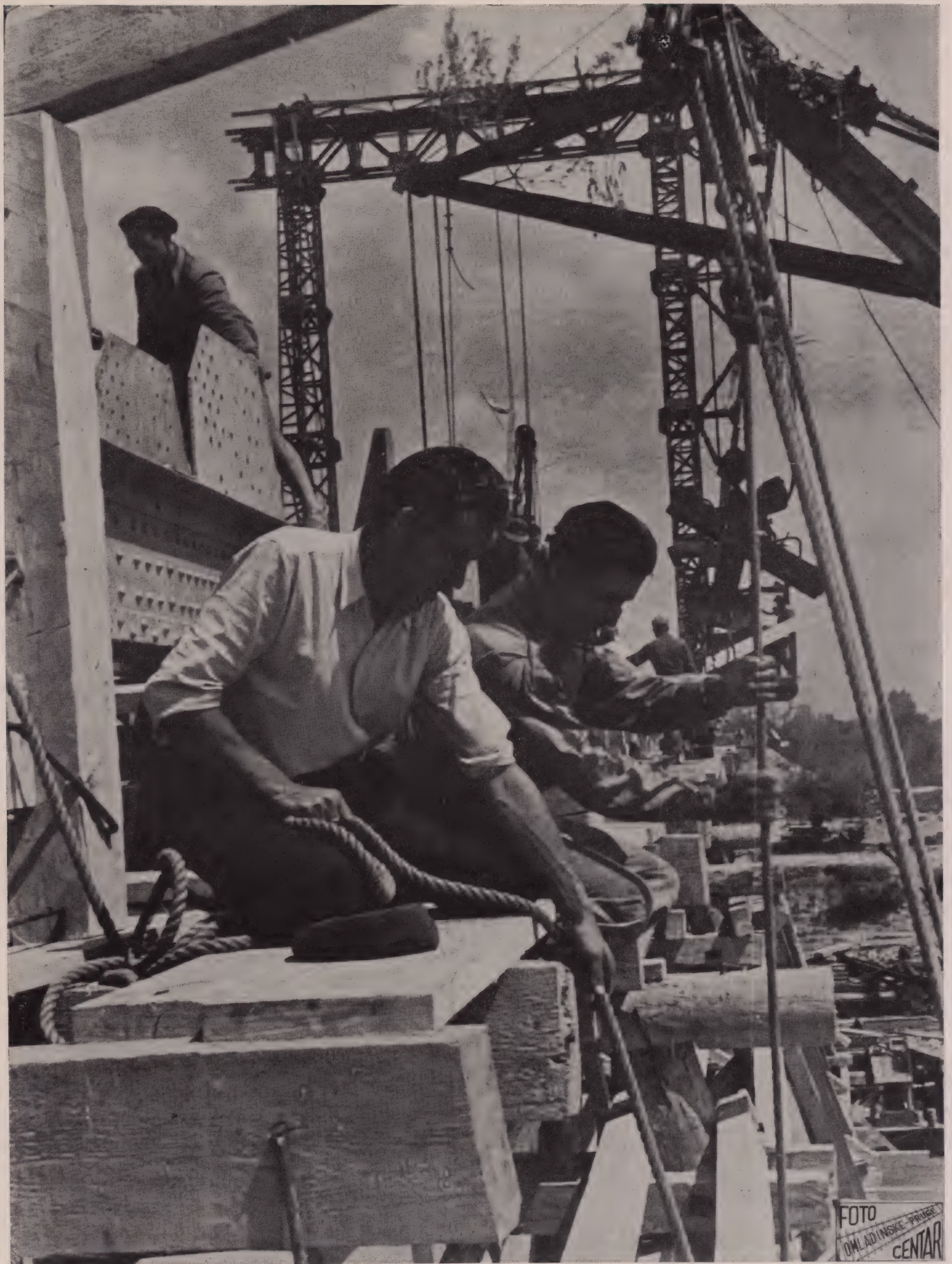
BRIDGE BUILDING WAS all in the day's work in putting through the Samac-Sarajevo Railroad line, completed in November.
