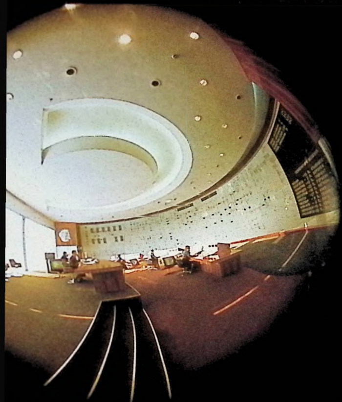
central control room of the Integrated Power Plant of the USSR. The grid makes it possible to efficiently channel the energy generated by the dozens of power plants in the country. Below: A module of the experimental installation devised by a research group at the Institute of High Energy Physics in Protvino, where a new fundamental particle was discovered.
