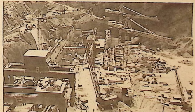
Full-speed construction guarantees early completion of new power center, which began generating in 1972.
