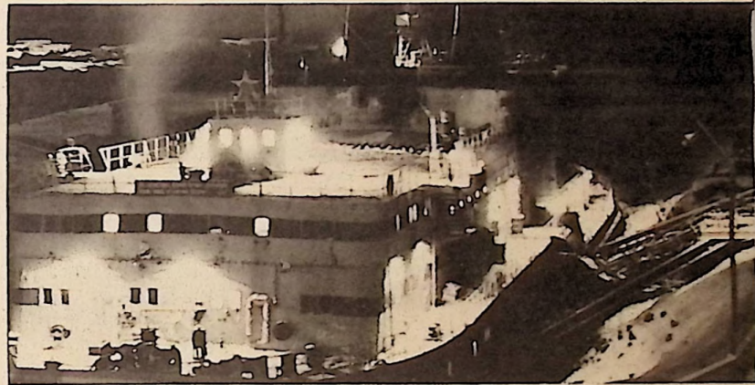
They're developing their Far North so fast that they can't wait for big power plants in all regions: so they're using floating generator stations like this "Northern Lights" ship. Burns diesel fuel and can power a large town. It's moored here on Kolyma River, having been brought there via Polar Sea navigation route.
